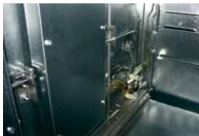
Interlock for circuit breaker compartment door
