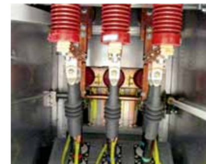
Connected power cable to the feeder busbar
